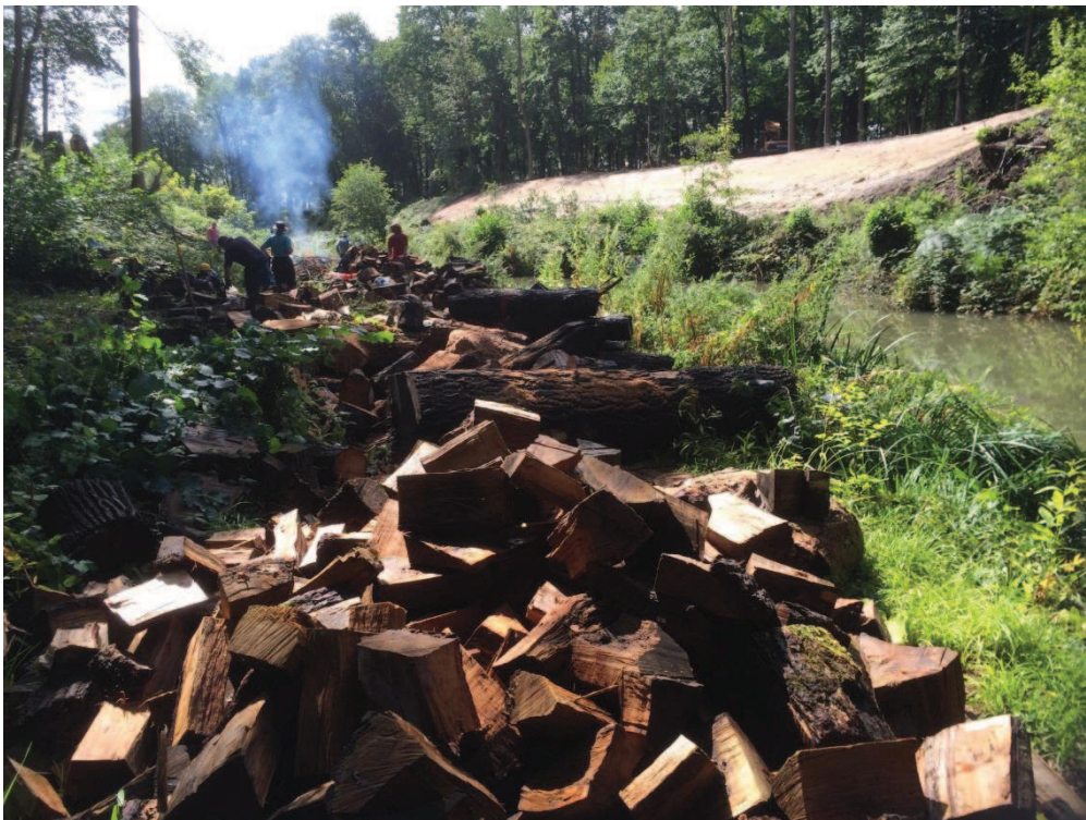
Removal of logs from the Dogmersfield landslip
